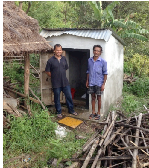
A beneficiary stands with the team leader next to his family’s newly constructed latrine
